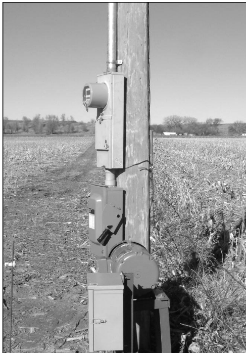
If you have an irrigated field with a center pivot and there is a single-phase power line close, then you too can enjoy the benefits of having electricity operate your pivot.
